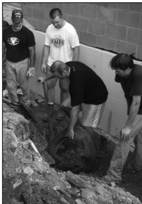
Attorneys Mitchell Shahan (from left), Leo Bouwers, Garen Fedeles and Garrett Harper remove debris from the home's foundation.
